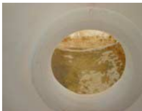
The inside of a water tank at a shepherd camp. The water in the tank was used by the worker for the purpose of cooking, bathing, and drinking. The tank emitted a rancid odor.
